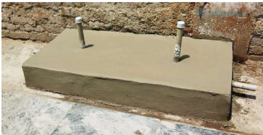
Fig 1.10 Reference Image of Pillar with the Meter Box Enclosure
